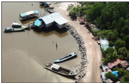
Figure 3. The revetment building with a dump stones system in Bandar Bakau Dumai (Source: Aras Mulyadi Personal Documentation Year 2020)
